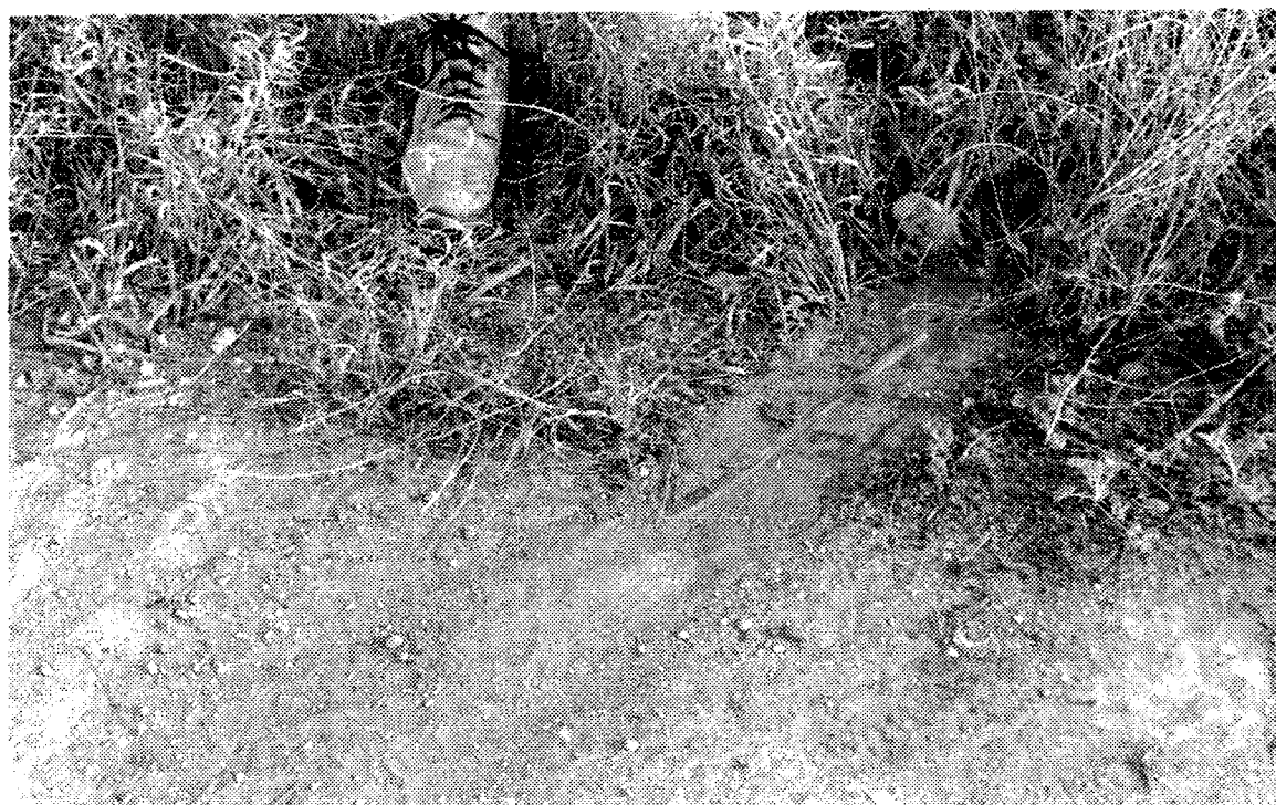
Figure 5.19 Rosthern brickyard site, concrete floor. with imbedded steel bar, bent and scraped.
