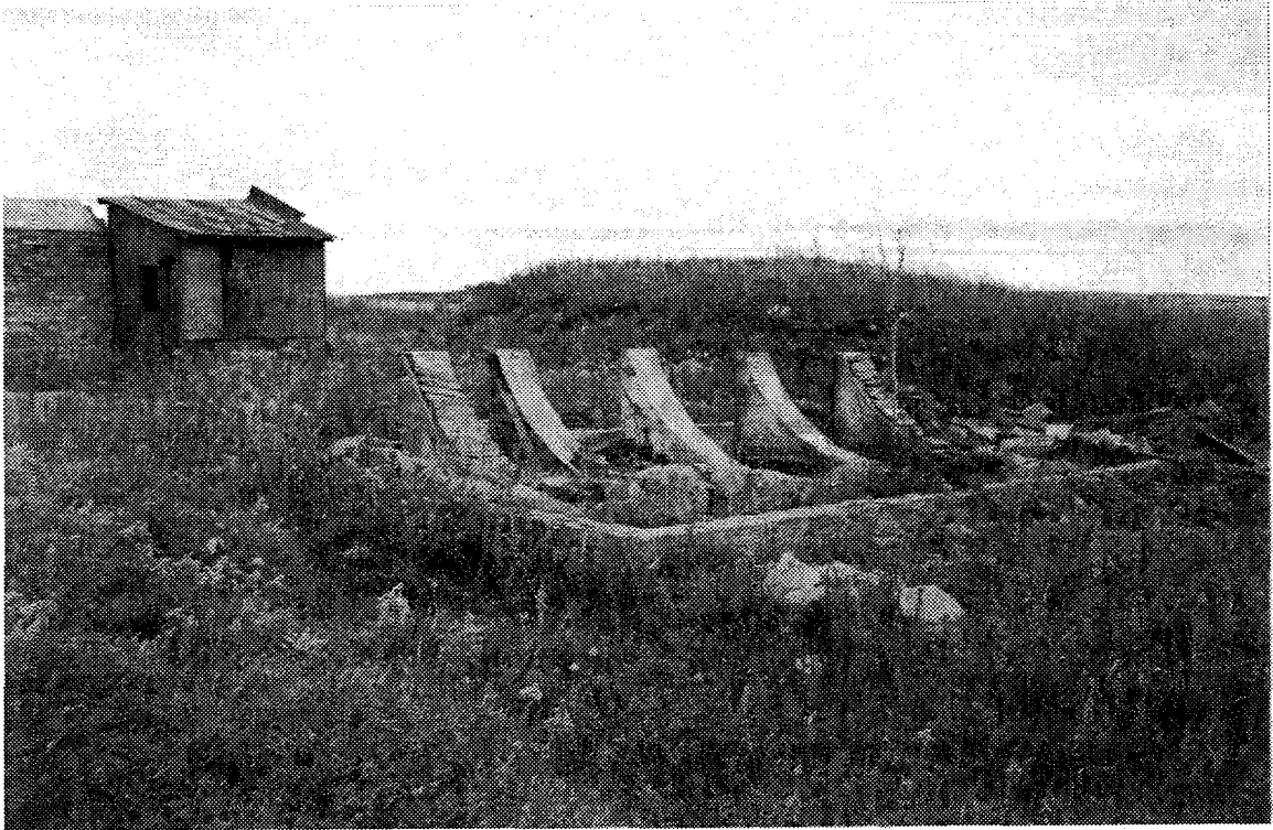
Figure 6.6 Bruno site in 1995: cradle for holding fuel oil tank for drying furnace.
