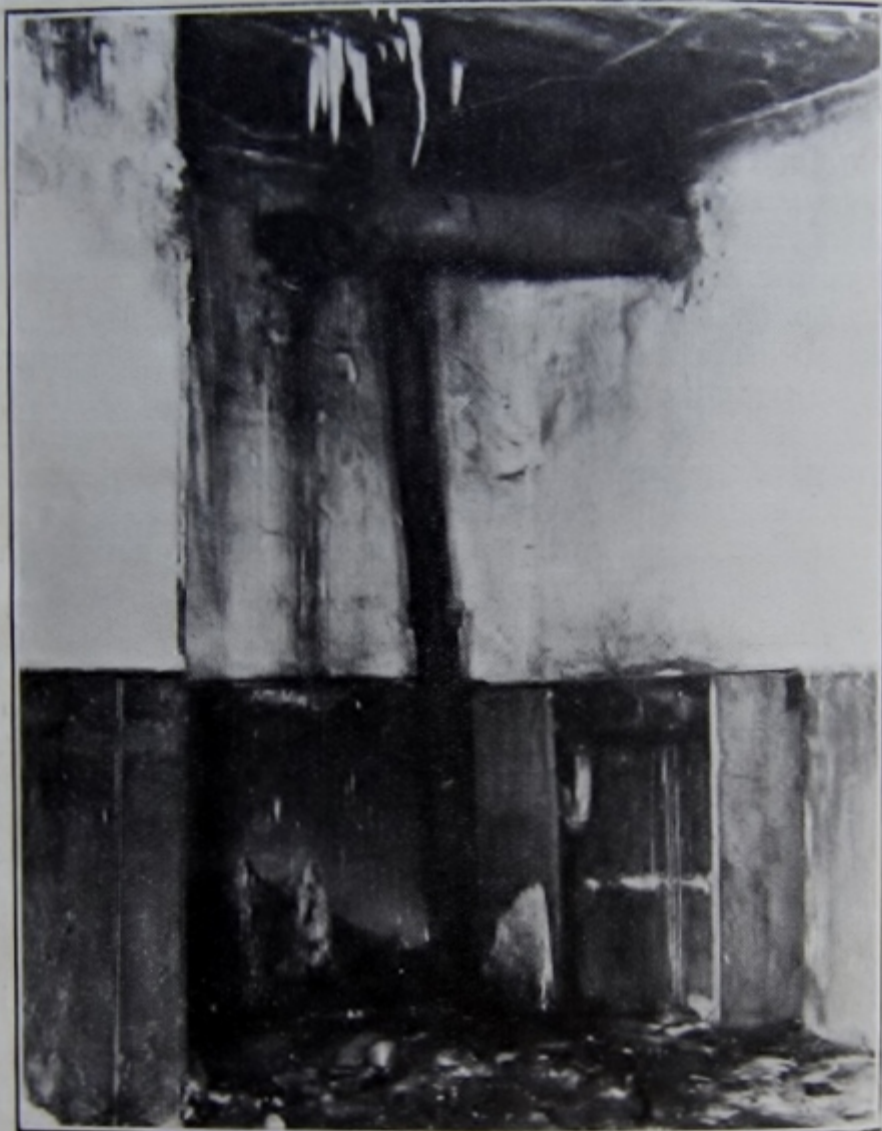
A Family of Twelve Occupied this Basement and Two Small Rooms. Note Icicles from Roof and Ice on Floor. Plumbing Bad.
