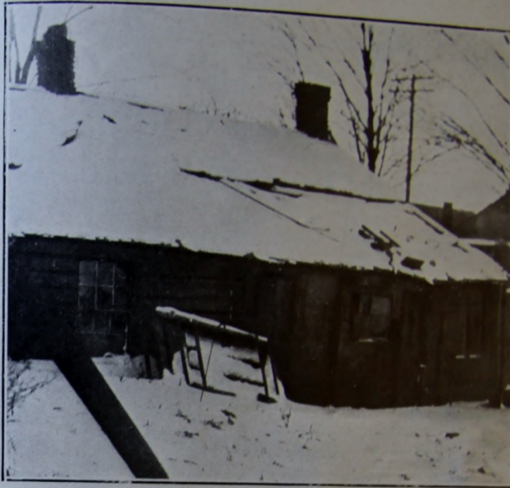
CLOSED BY HEALTH DEPARTMENT As Unfit for Habitation. A Small Bedroom, a Small Living Room. Six in the Family.
