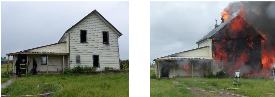
Figure 1.7 Prince Albert full scale fire test before (left) and during (right) fire experiment (Fulton, et al. 2017b)
