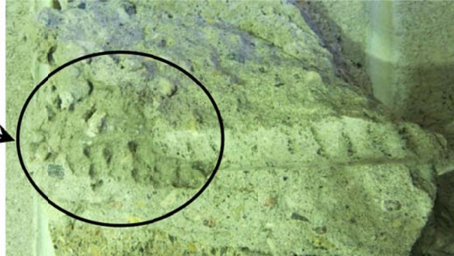
Figure 4.7: Inadequate Grout Consolidation Around the Longitudinal Reinforcing Bar in the Splice Region of the NCLS#3 Wall Splice Specimen.
