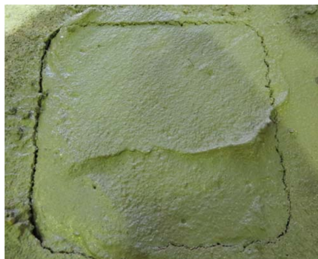
Figure 2.10: Shrinkage Cracks at the Grout-Block Interface.
