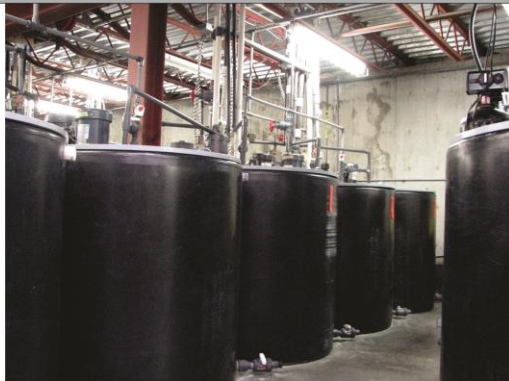
Figure 6. View of grow tanks in the seedling wing and nutrient-brine supply tanks in the basement of AAFC's Salinity Lab.
