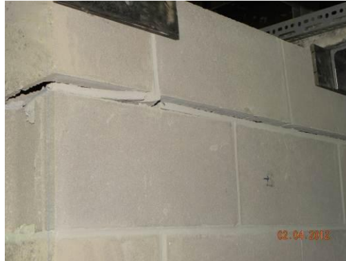
Figure 4.19: Crack formation from unloading of the wall
