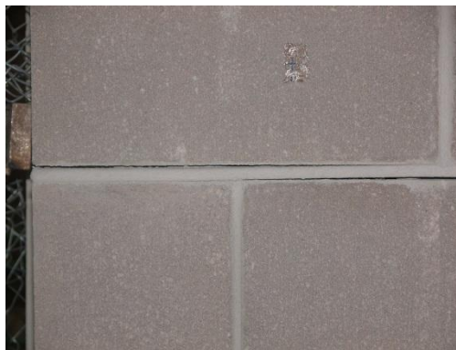
Figure 4.11: Typical cracking pattern for all wall specimens
