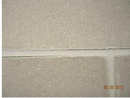
Figure 4.13: Cracking of wall prior to testing
