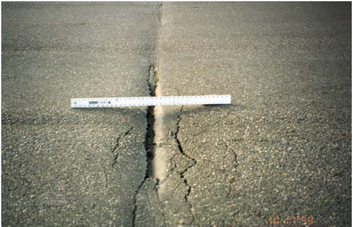
Figure 2.3 Thermal Crack Depression in Asphalt Concrete
