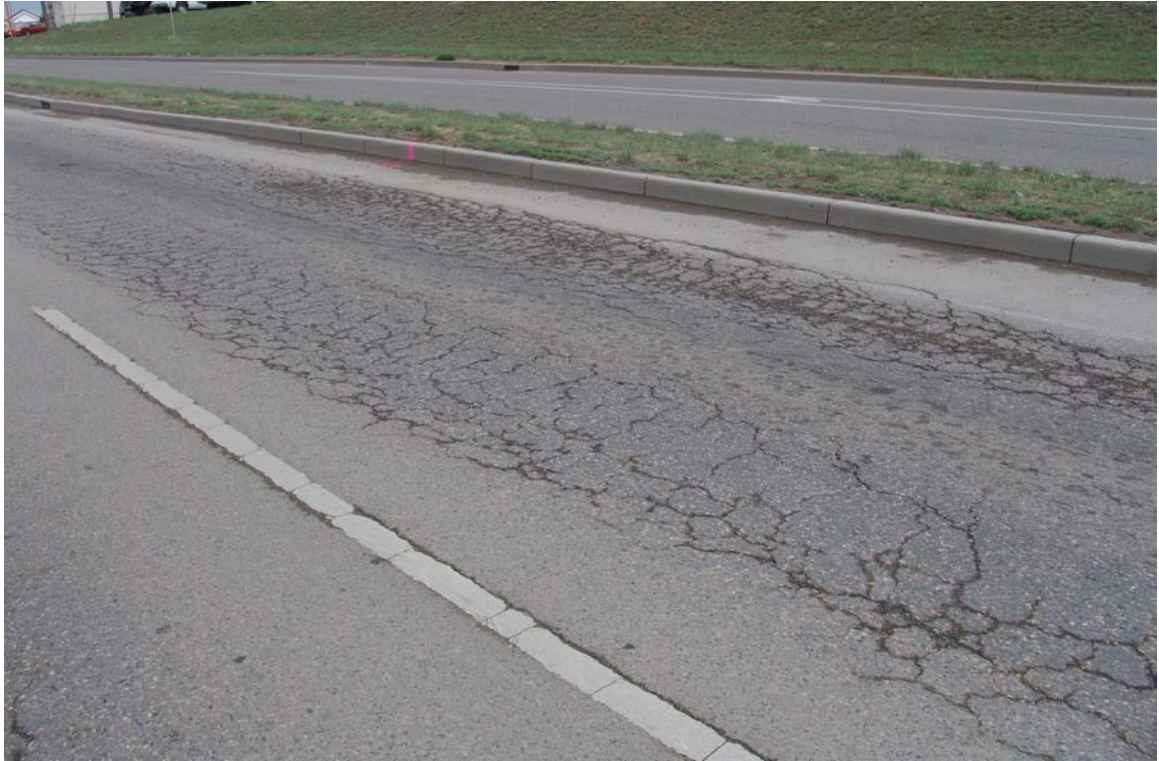
Figure 2.5 Substructure Rutting with Fatigue Cracking
