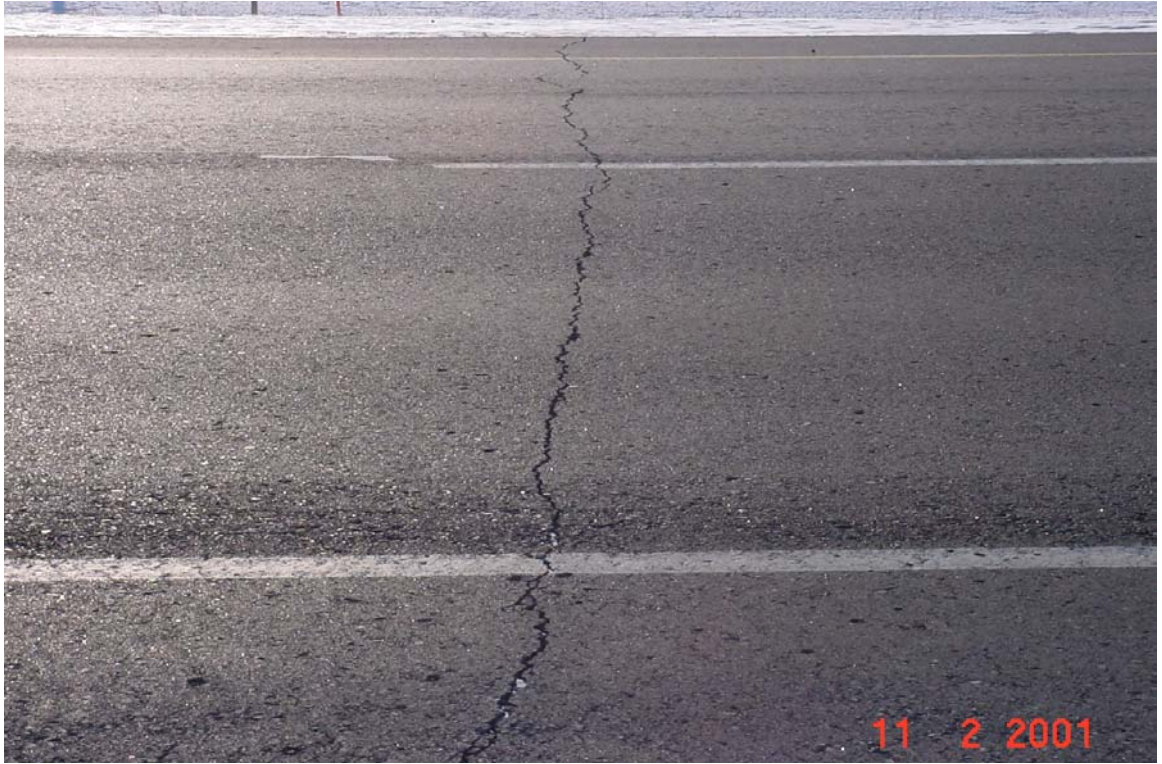
Figure 2.2 Thermal Cracking in Asphalt Concrete
