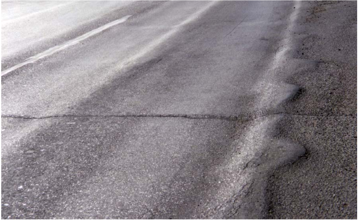
Figure 2.7 Asphalt Concrete Layer Viscoplastic Rutting
