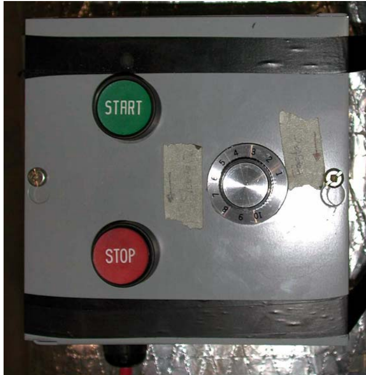
Figure F.15: Pump motor variable frequency drive (VFD) pot used in the 156.7 mm flume experiments
