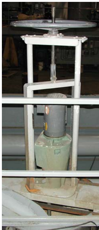
Figure F.26: Baldor mixer in the 156.7 mm flume circuit stand tank
