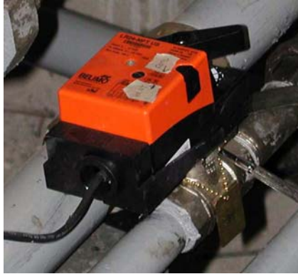
Figure F.17: Belimo control valve on the glycol-water fluid heat exchanger line used to control the system temperature in the 53 mm feed pipe used in the 156.7 mm flume experiments
