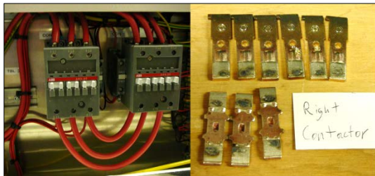
IMAGE 2. RF power distribution contactors (left) and their pitted contact surfaces (right).
