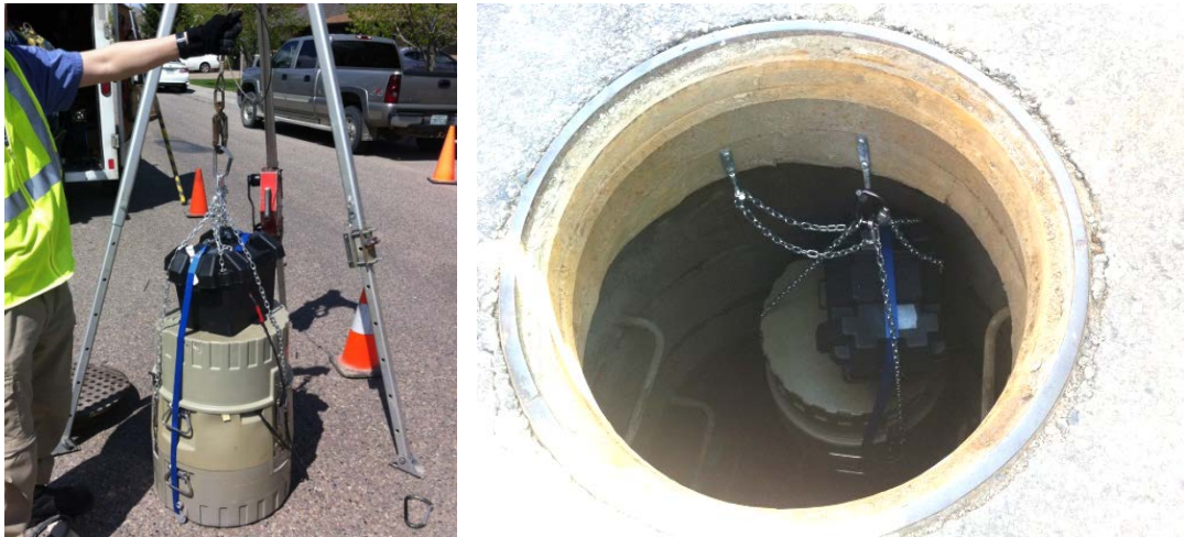
Figure 3-9. (Left) ISCO samplers and batteries with tie strap and chain assembly hung in manholes for easy retrieval (right).
