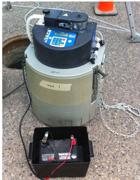
Figure 3-3. An ISCO 6712 series automated stormwater sampler with 12 V battery attached.
