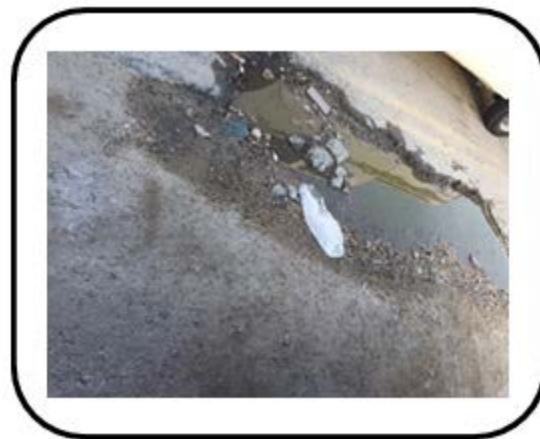
Figure 4.20. The street surface is not good for walking. Provided by Photovoice Participant 1.
