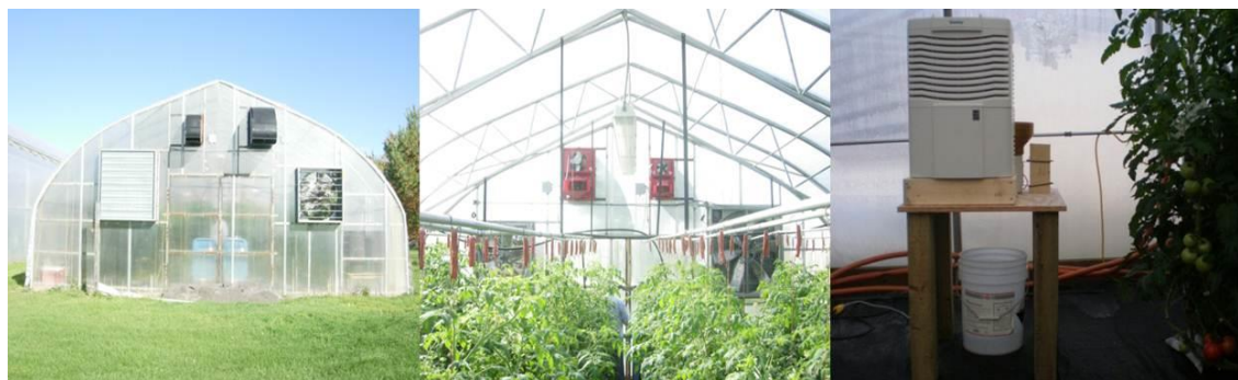
Figure 1.3. Heat exchangers (left, visible from the outside; center, visible from the inside) and Model 6510E dehumidifiers setup (right).
