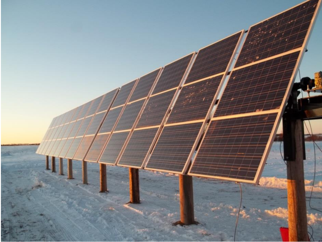
Figure 2.4: 8.19 kW Solar Array [49]
