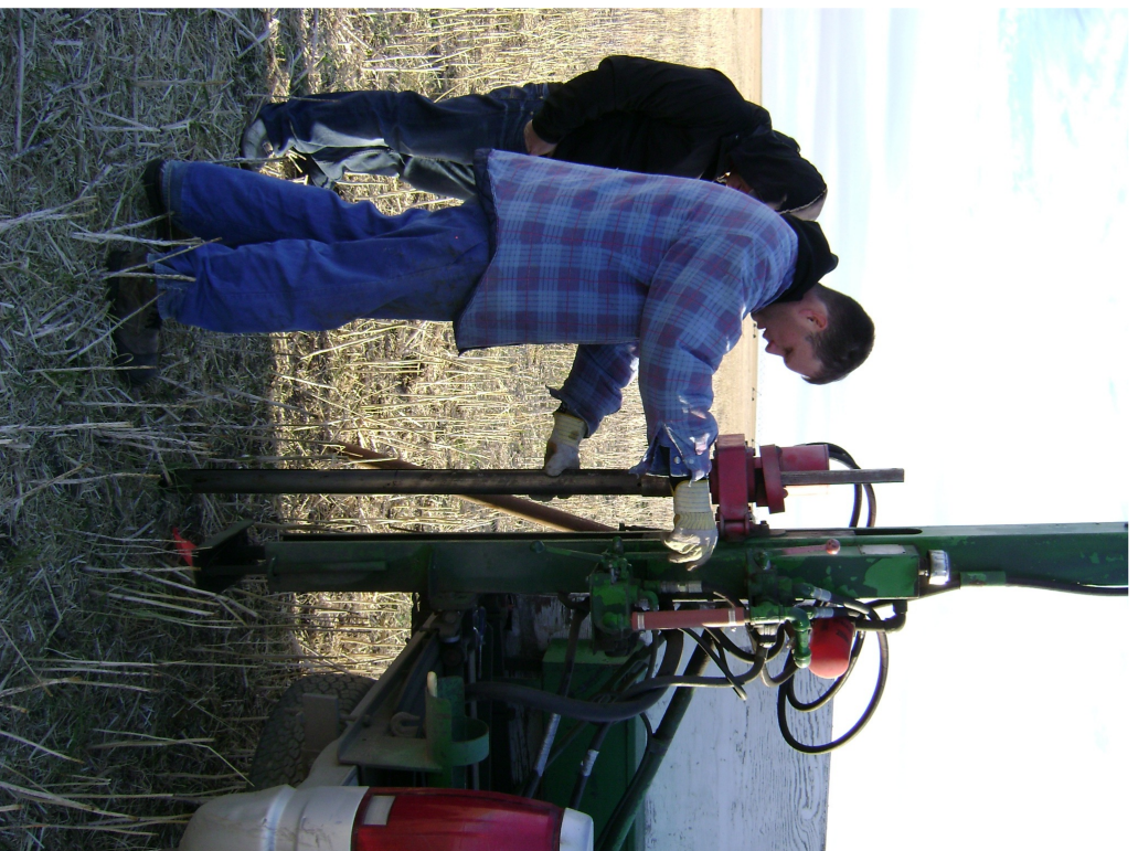
Fig. A7. Cory Fatteicher extracting soil extracting soil core with a truck mounted punch
