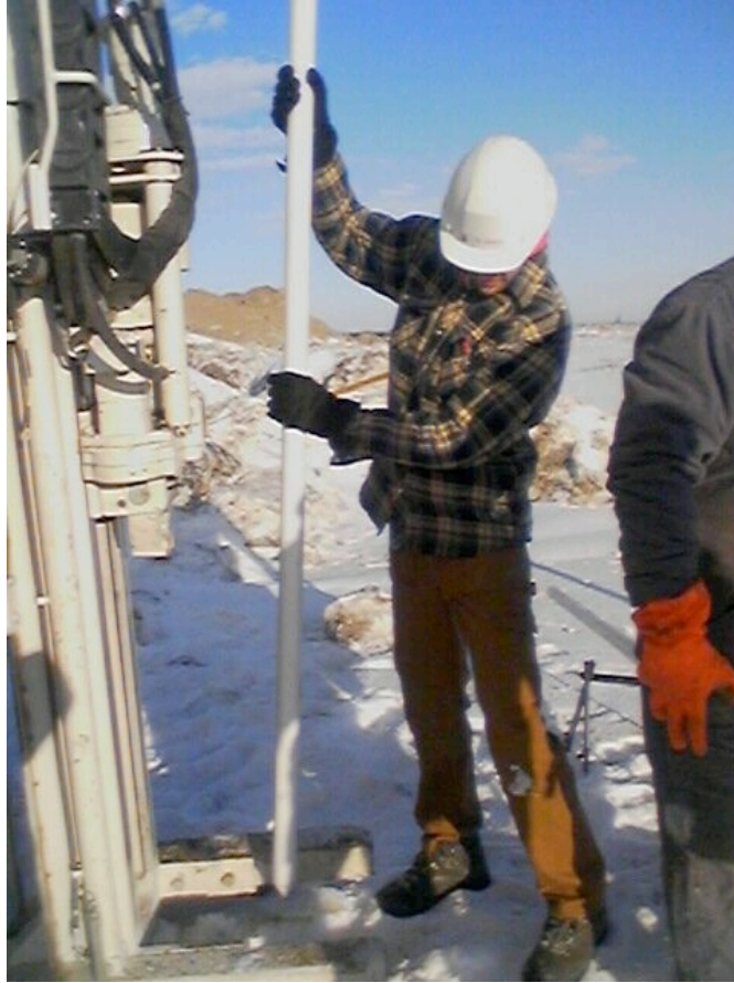
Figure 3.4 - Installation of ES and Deep Diviner access tubes using the CPT rig. In this photo, the larger 83 mm casing is being installed following sample coring.
