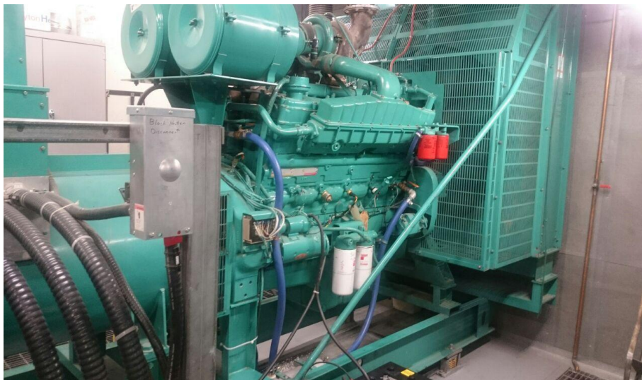
Figure 5.5 Diesel generator at SPH.
