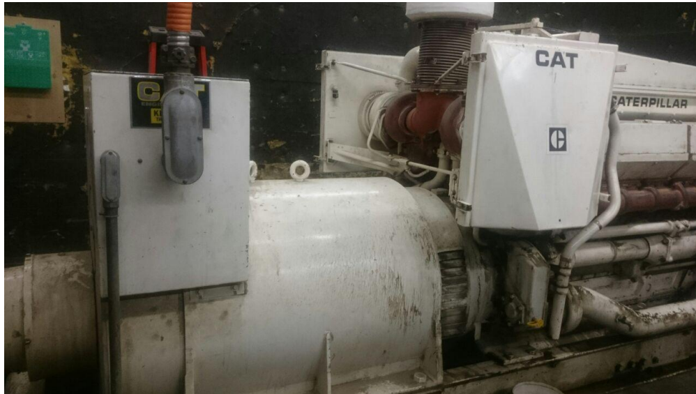
Figure 5.1 Diesel generator at RUH.
