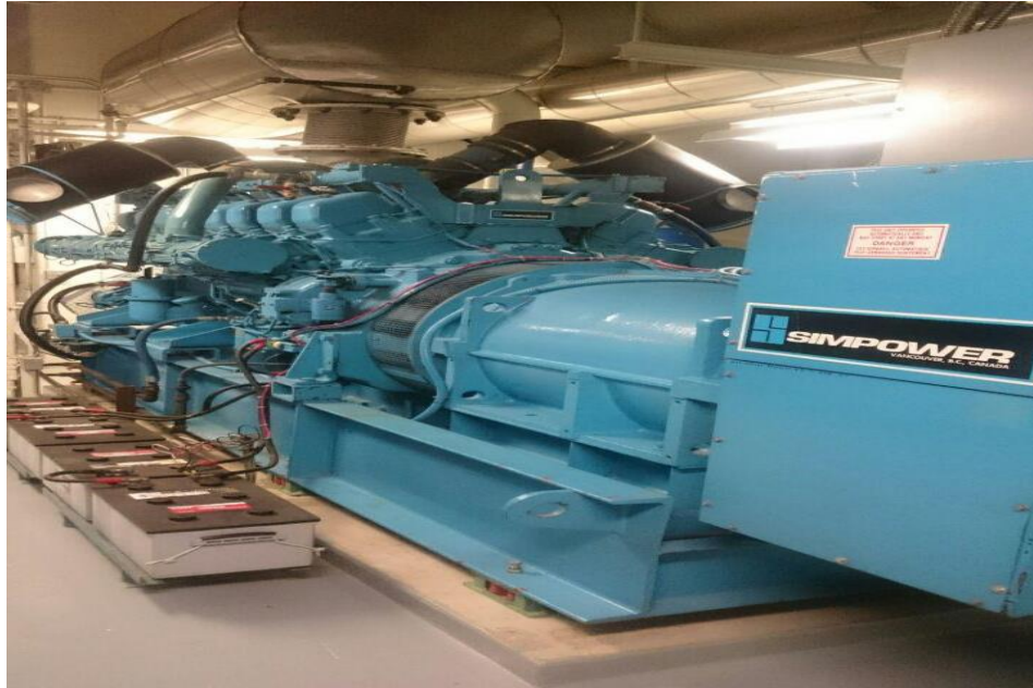
Figure 5.3 Diesel generator at SCH.
