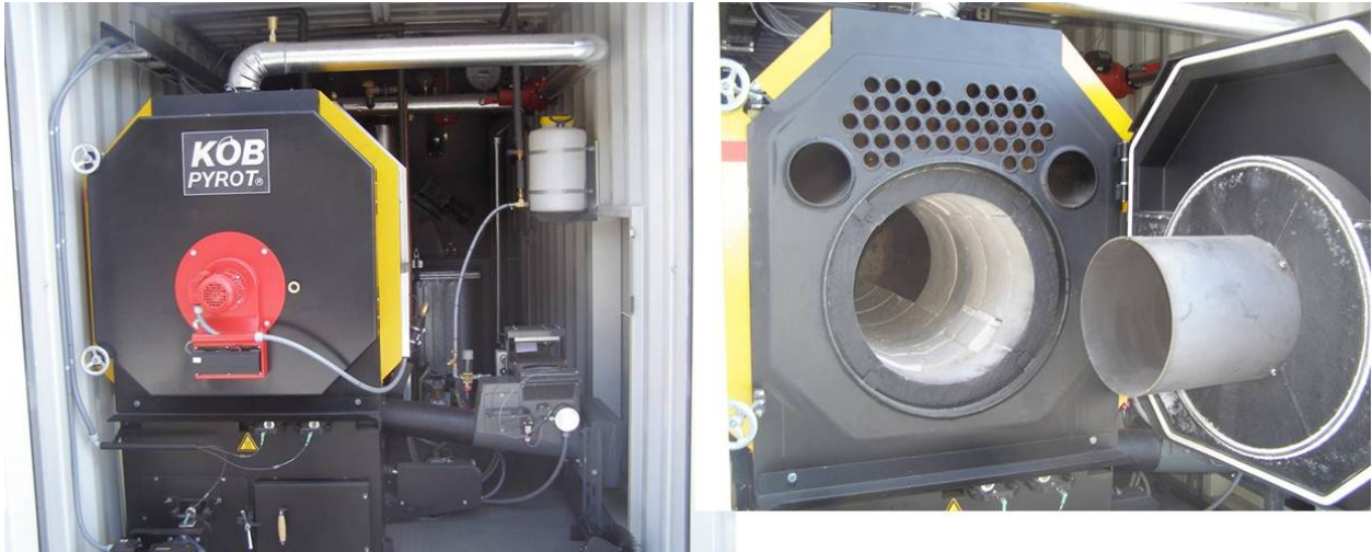
Figure 8. The KOB Pyrot combustion biomass boiler located at the ADC in Indian Head, SK.
