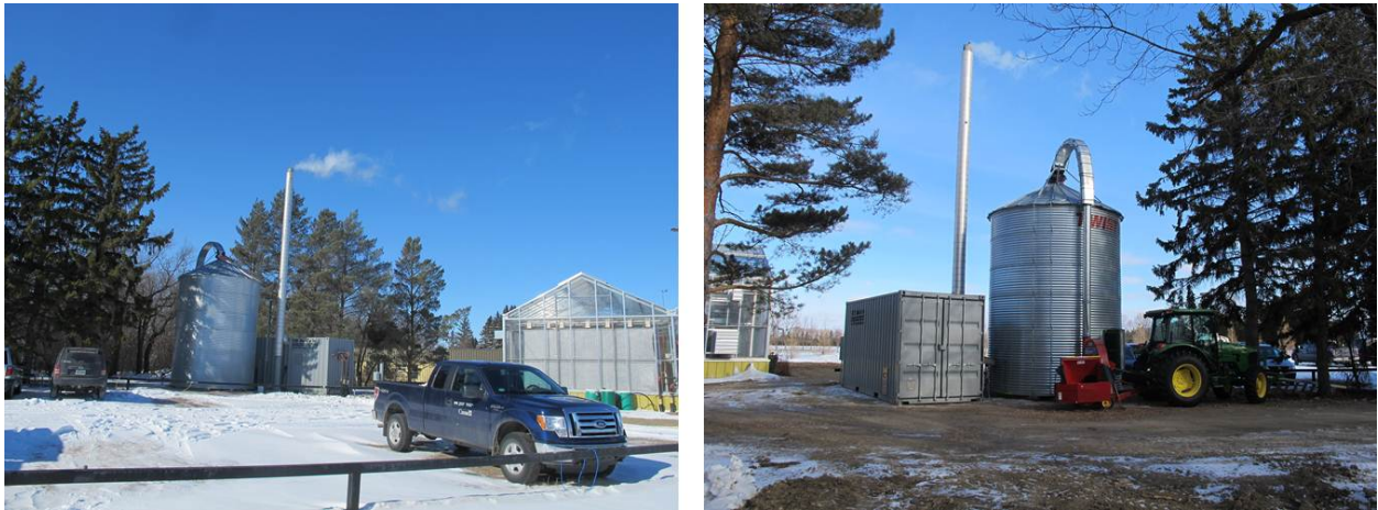
Figure 9. The biomass heating system in operation at the ADC in Indian Head, SK.
