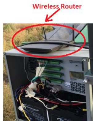
Figure 2-59: Utilized Wireless router
