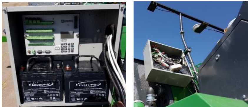
Figure 2-48: Utilized datalogger inside a control panel
