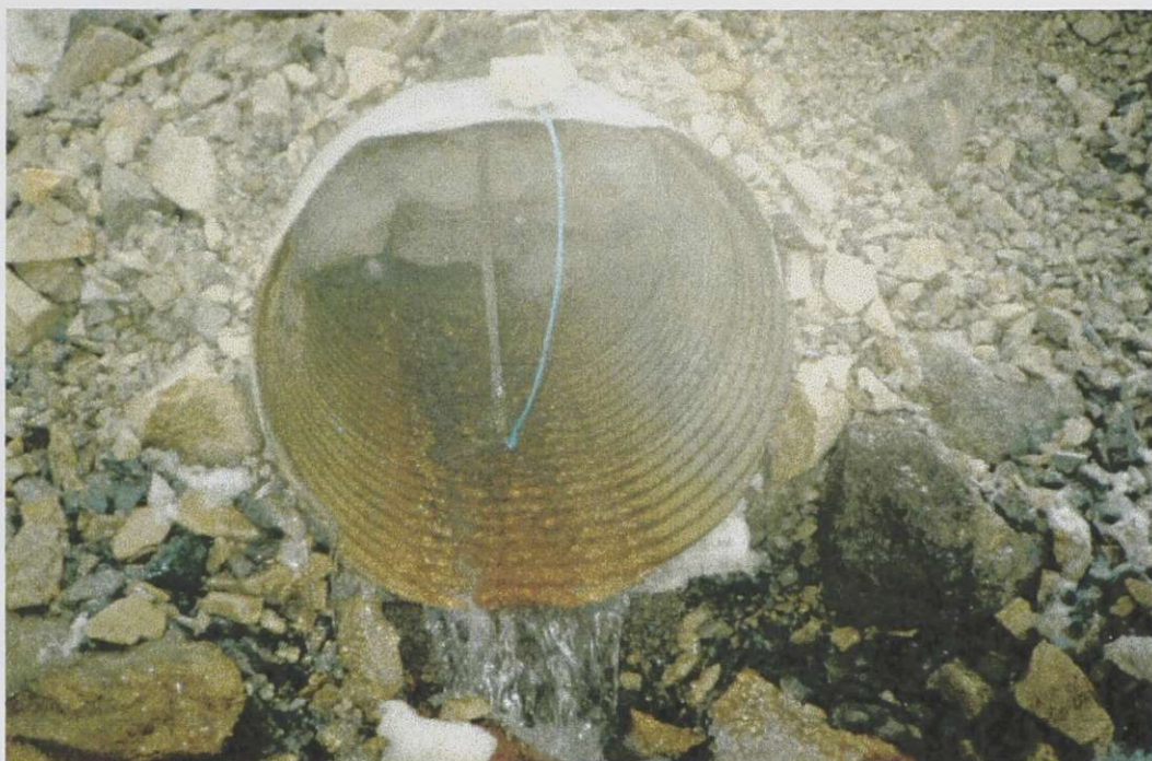
Figure 4.10 Culvert flow instrumentation (R 98-01 station).
