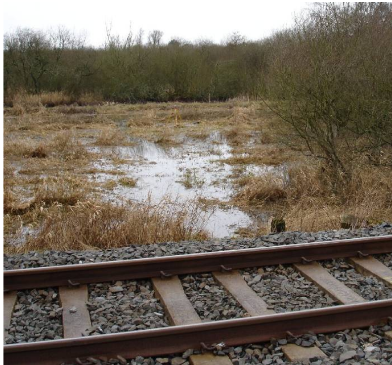
Figure 1.2: Embankment at Brackagh bog with surrounding area flooded during winter months
