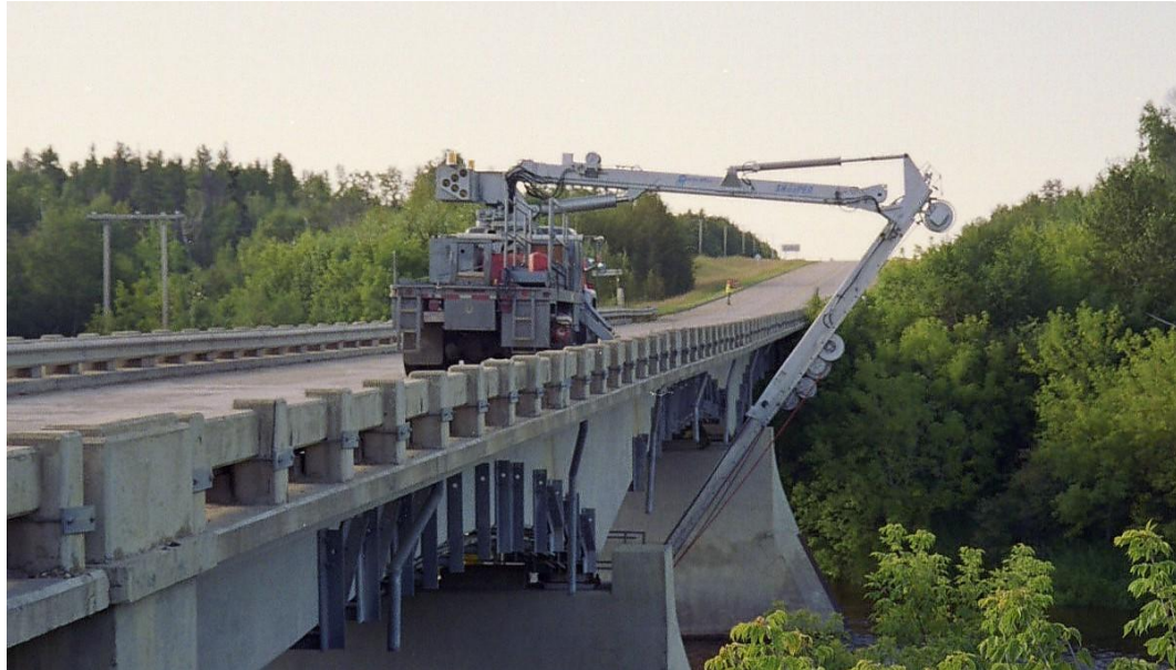
Figure 3.8 Snooper truck used to install the strain gauges on Hudson Bay bridge.
