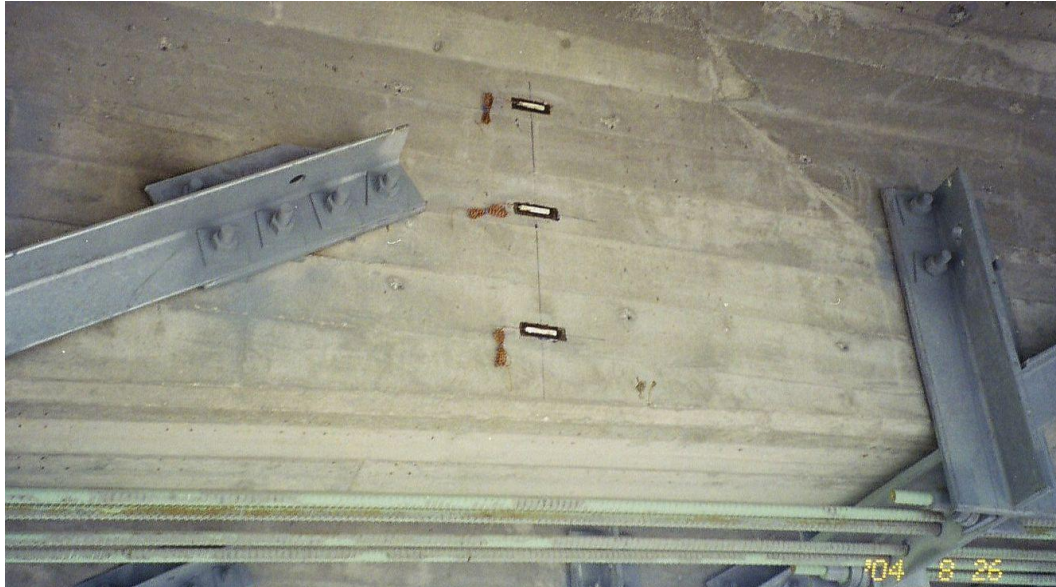
Figure 3.7. A group of strain gauges as installed on Hudson Bay bridge.
