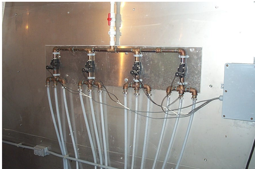
Figure 5 Solenoid valves in washing gutter chamber.
