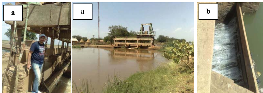
Figure A.1-4. Basatna barrage (a) and the outlet is controlled by wood sheet (b)
