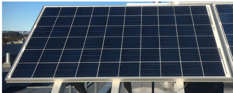
Figure 18 – Picture of one of the solar panels used
