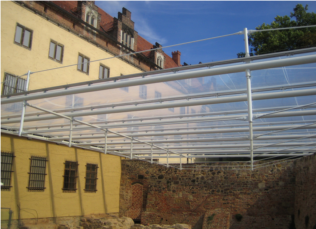
Figure 2.16: Lutherhaus, Germany (2010) . Pressurised transparent foil cushions supported by cable supported steel beams.
