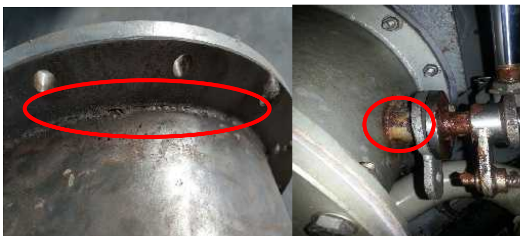
Figure 1.5: Area of Crack at Exhaust Heat Exchanger
