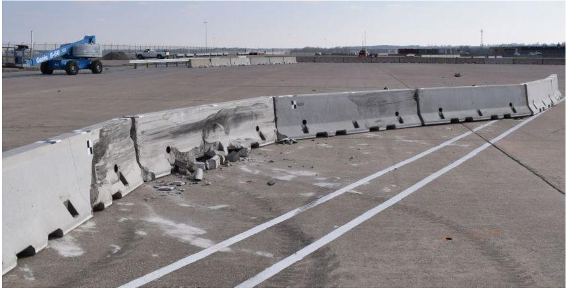
Figure 73. System Deflection and Damage, Test No. NELON-1
