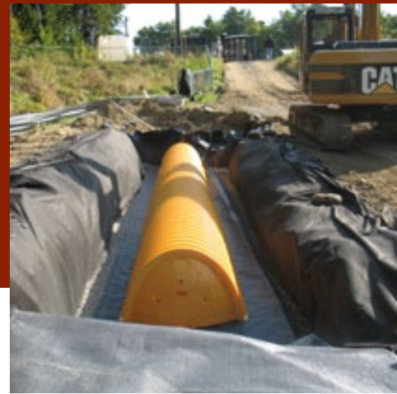
StormTech Isolator Row.
