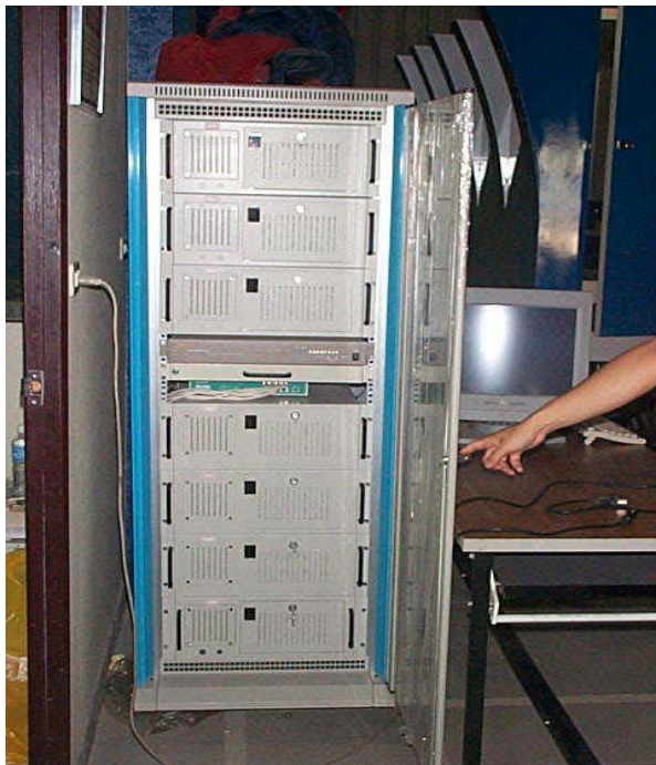
Figure 13. Rack-mounted computers to form a COP
