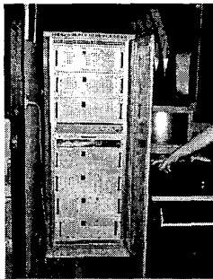
Figure 11. Rack-mounted computers to form a COD
