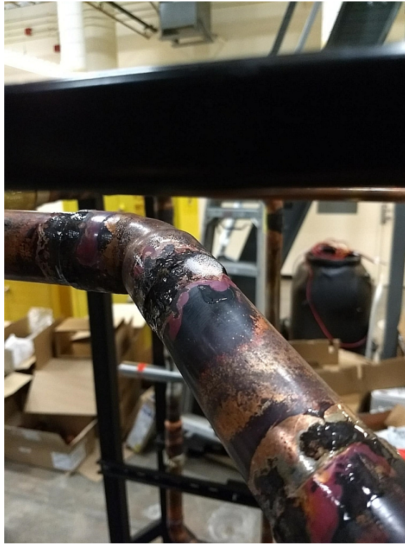
Figure 5.14: Formation of bubble colony due to small leak in brazed joint
