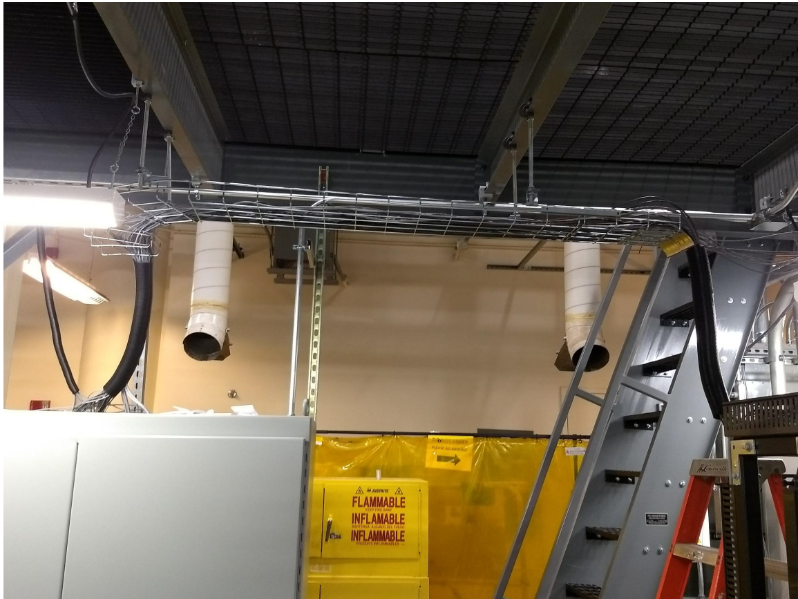
Figure 6.4: Wiring from the load stand following the suspended cable tray to the DAQ enclosure
