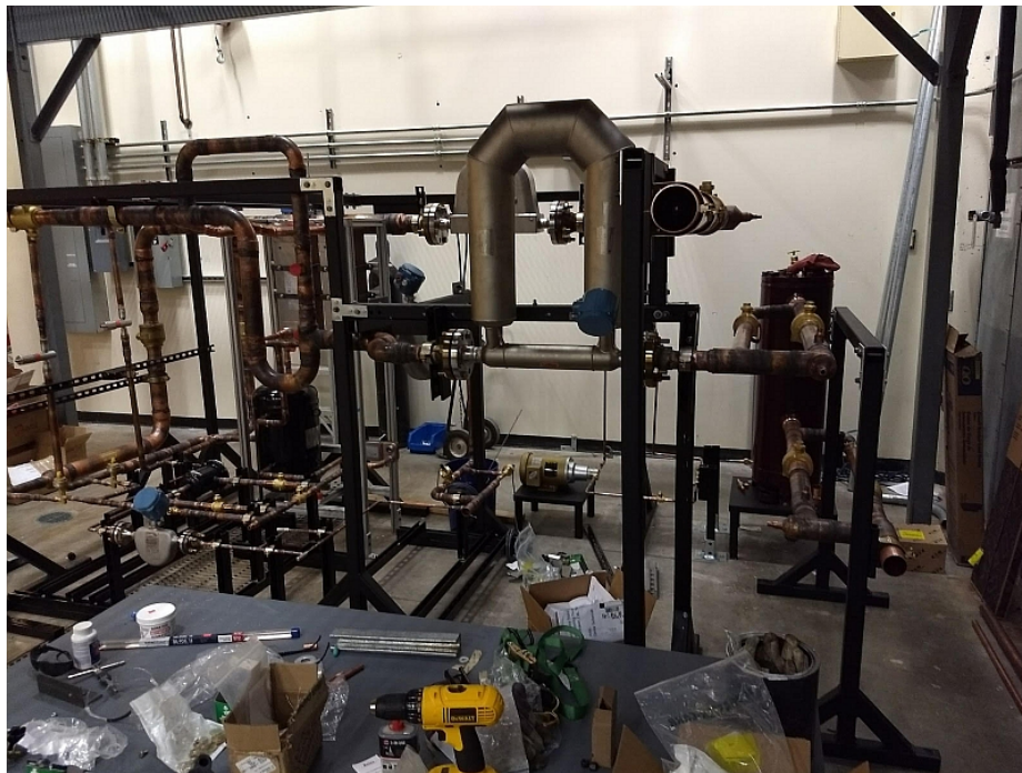
Figure 5.12: Most tube assembly completed and showcasing the parallel discharge tubing (right) required due to high pressure requirements.
