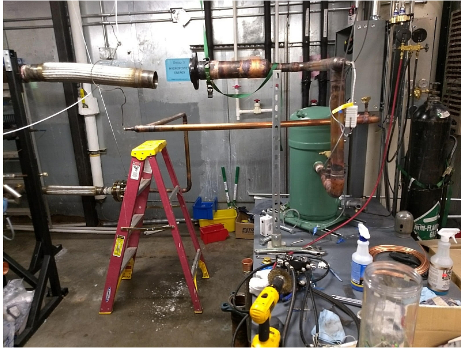
Figure 5.13: Compressor manifold assembly with the suction line flange connection incomplete.
