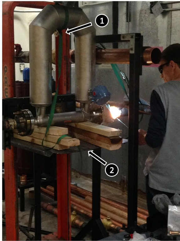
Figure 5.11: Undergraduate research assistant Jake Singleton brazing discharge mass flow meter in place with the help of ratchet straps (1) and the presto lift (2).
