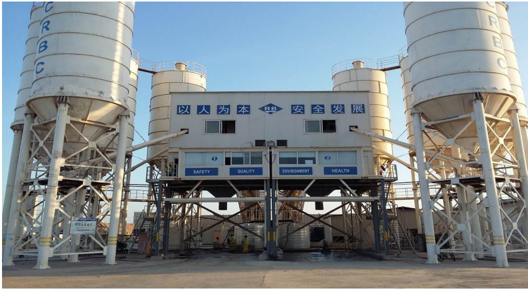
Fig.4.3 – South Bank computerized batching plant
