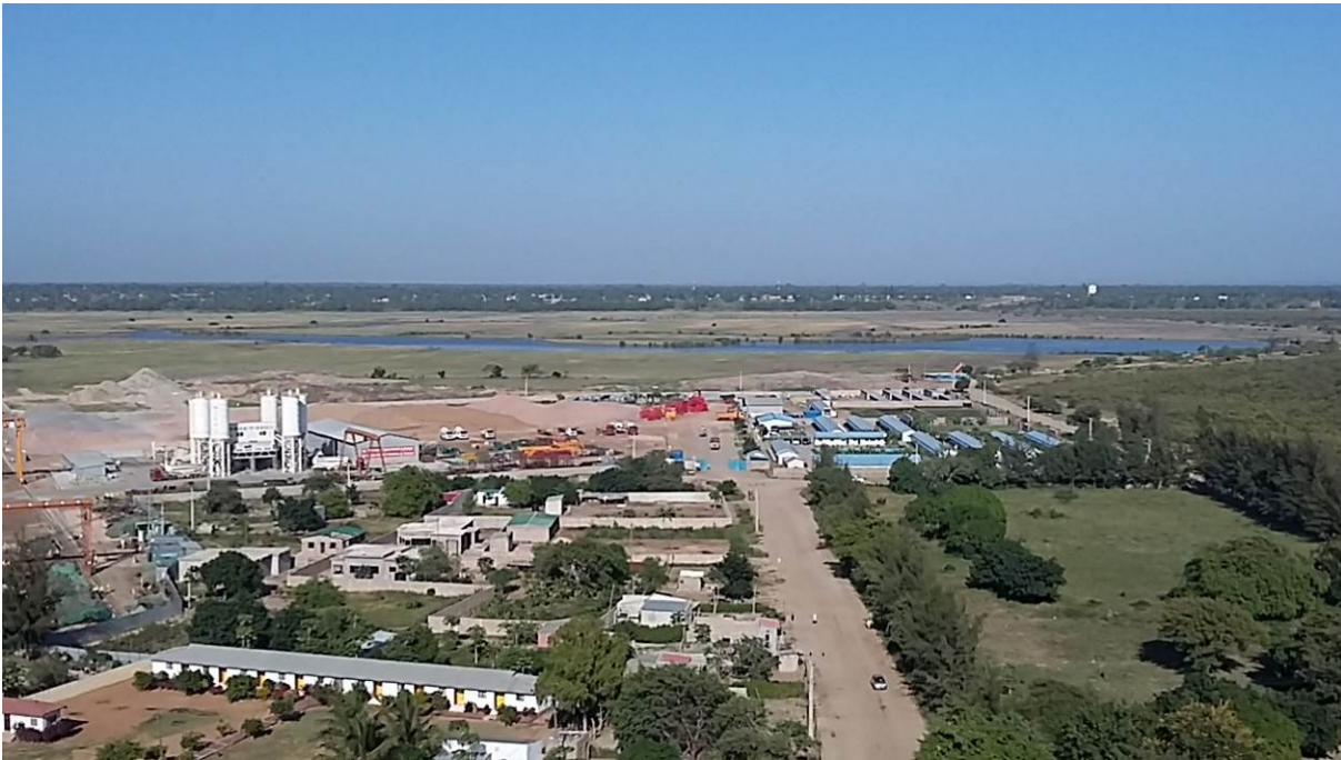
Fig.4.1 – View from Pylon M2 with the site entrance, the batching plant on the left and the Chinese camp on the right
