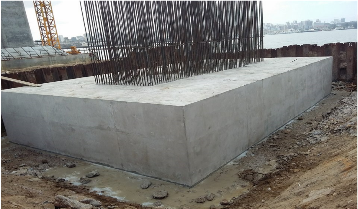
Fig.5.2 – Pile Cap S1 before backfilling and with the starter bars for the first layer of pier body reinforcement
