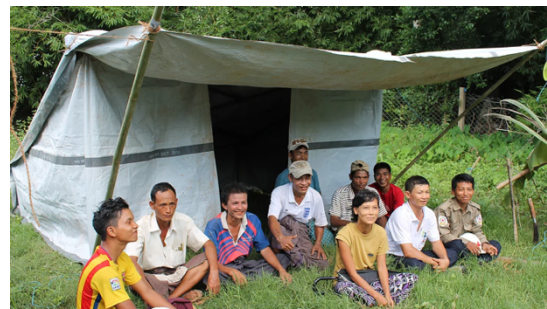
Figure 101 - Red Cross and villagers in Myanmar Delta build emergency RSK shelters 2017 (RSK Shelter 2018)
