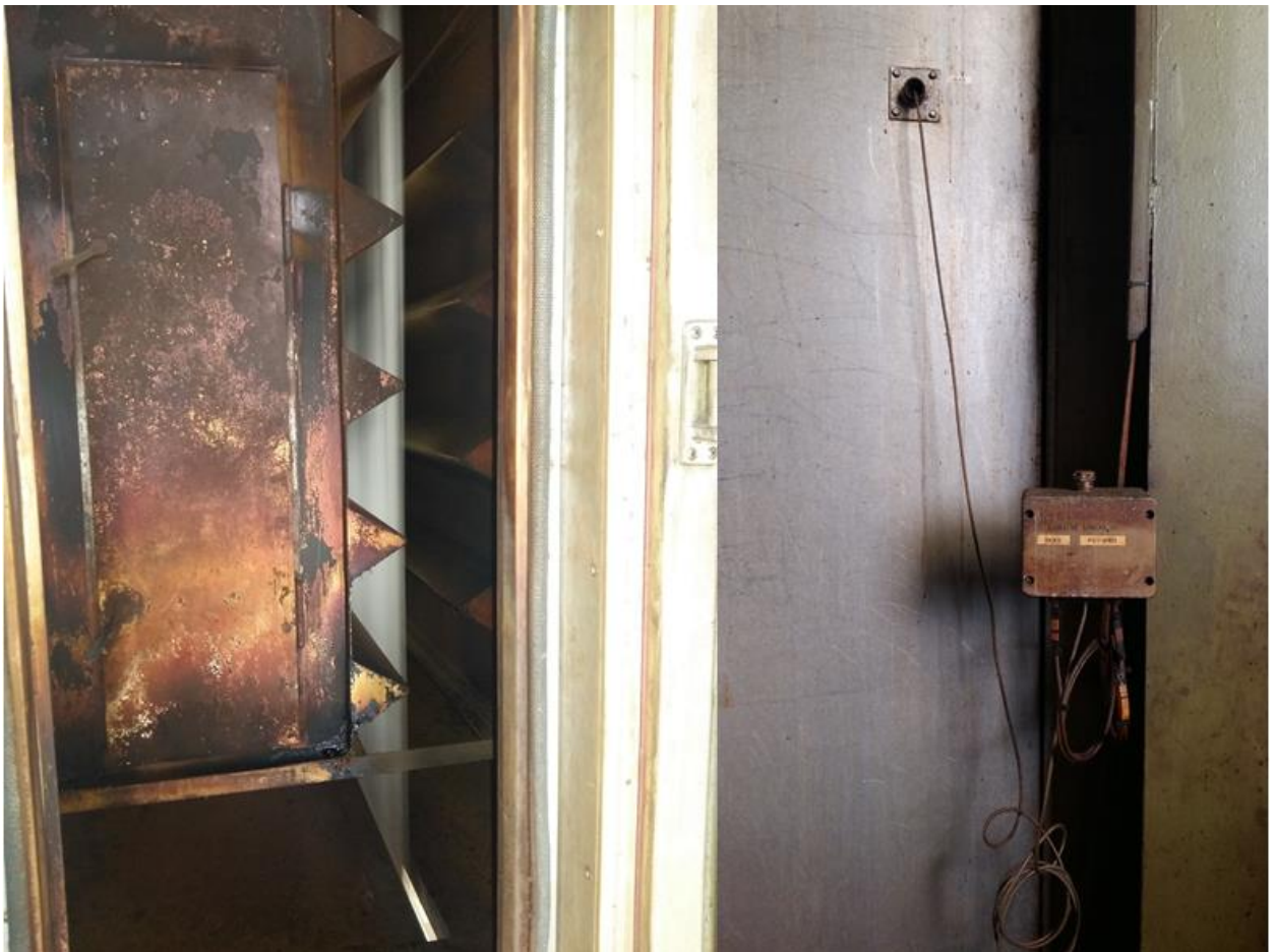
Figure 37. Inside view of the Oven 5 with the jet boxes and fabric on movement and one of the temperature measure device.
