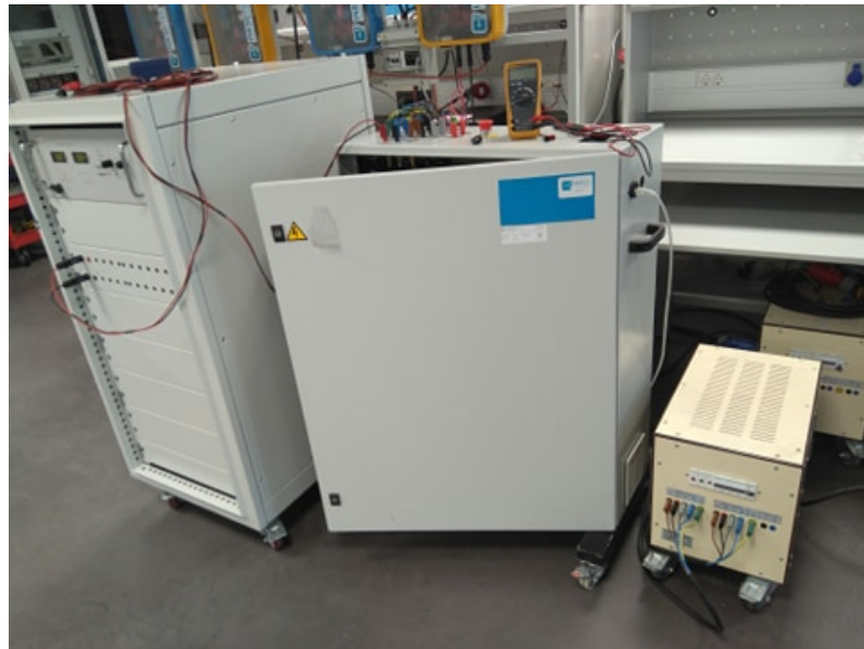
Figure 5.6: DC Source (left), inverter (middle) and transformer (right)
