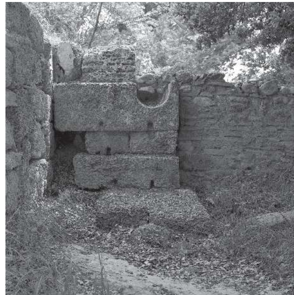
Fig. 4 Retaining wall of the western stadium embankment (left) with water channel in the front and a later wall cutting the channel (right).
