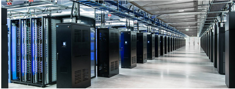
Figure 1.3: An interior of a data center facility [6]
