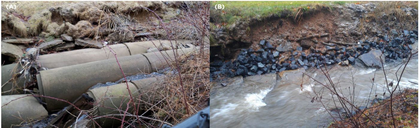
Culverts (A) were visually assessed to be impeding fish passage in the brook and culvert removal (B) restored habitat connectivity.
