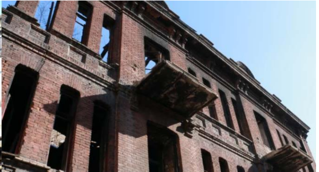
Figure 8. Only the old facade was left after the fire
