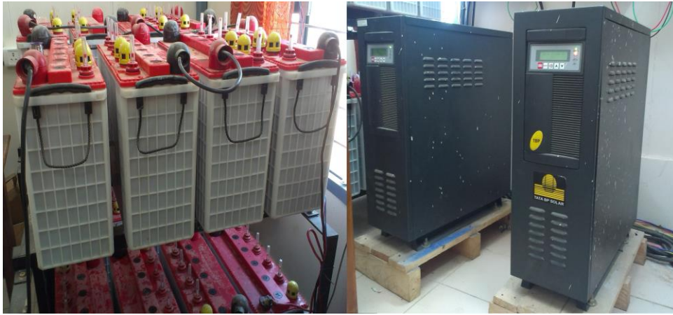
Fig.5.4 Lead acid batteries with charge controllers
