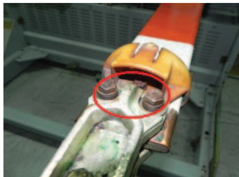
Fig. 1: Corrosion and greenish stain on the switchgear part.
