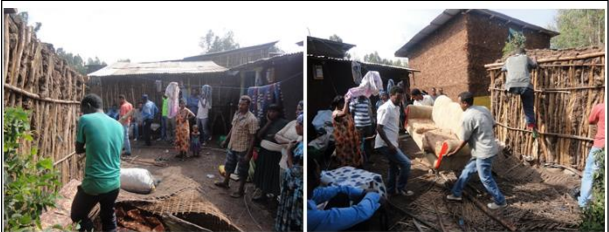
Figure 6.7: Some of the demolishing team (left) and unauthorized buildings after demolition (right)
