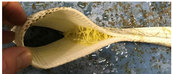
Fig. 9. Sample 1-TTS. Belt loop failure. Complete failure at headstock end (upper picture) and partial failure at tailstock end (lower picture).
