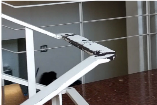
(a) Handrail in the Barcelona School of Architecture, in the landing between two flights of stairs. Generations of students grabbing the horizontal section to make a 180 degree turn have chipped part of the white paint away, exposing the metal.
