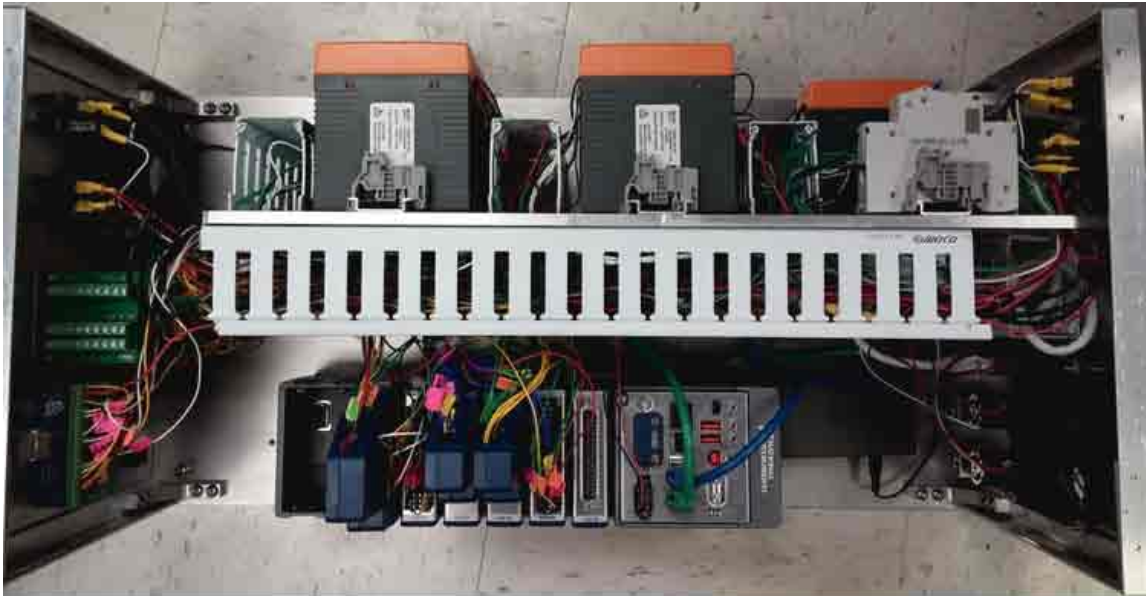
Figure 5.1: The inside of Control box. Control box consists of NI cRIO, ethernet hub, power supply, safety devices, and others. For the connections in Control box, screw-type breakout boards were used for convenient maintenance, and for the connection to the other peripherals, standard connector housings (D-sub 25/37, HDMI A-type) were used for quick and robust connections. The wires in Control box were cleanly arranged by Din rail, wire duct, terminal block, and label.
