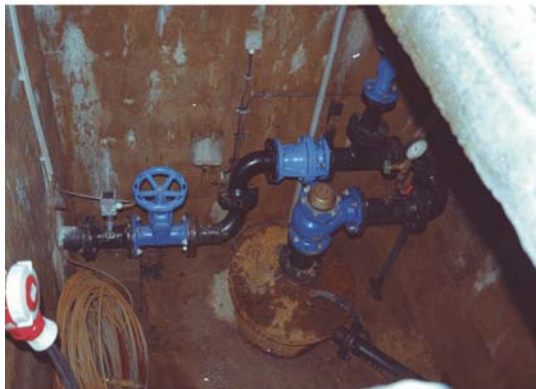
Brunnenstube TB Wolfersdorf TW 1/61
