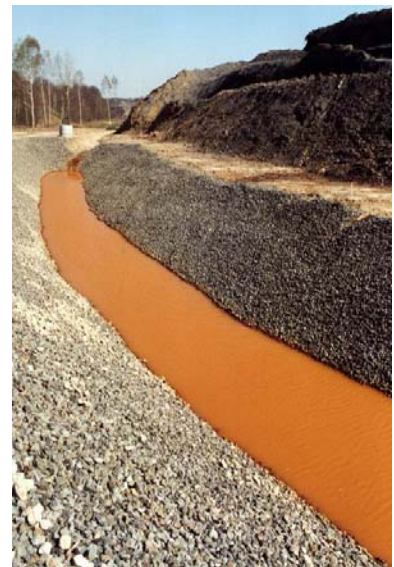
Figure 3: AMD collected in canals and pumped to a treatment plant. Photo: S. Senitz.
