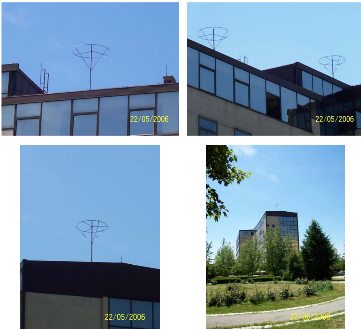
Fig. 5. Photos of installed lightning protection rod (JUS N. B4. 811).
