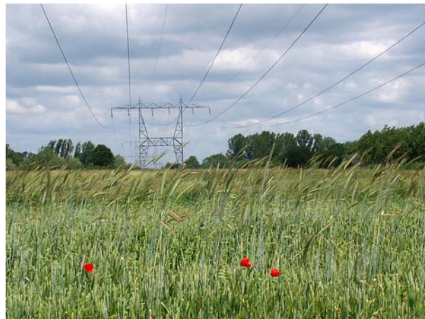
Fig. 2. 220 kV power line KLI – NIZ and 110 kV power line KLI – POL on common supports
