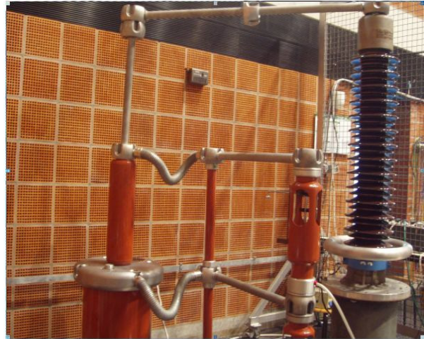
Figure 4: Test setup to simulate a partial breakdown by short circuit of a series capacitance.
